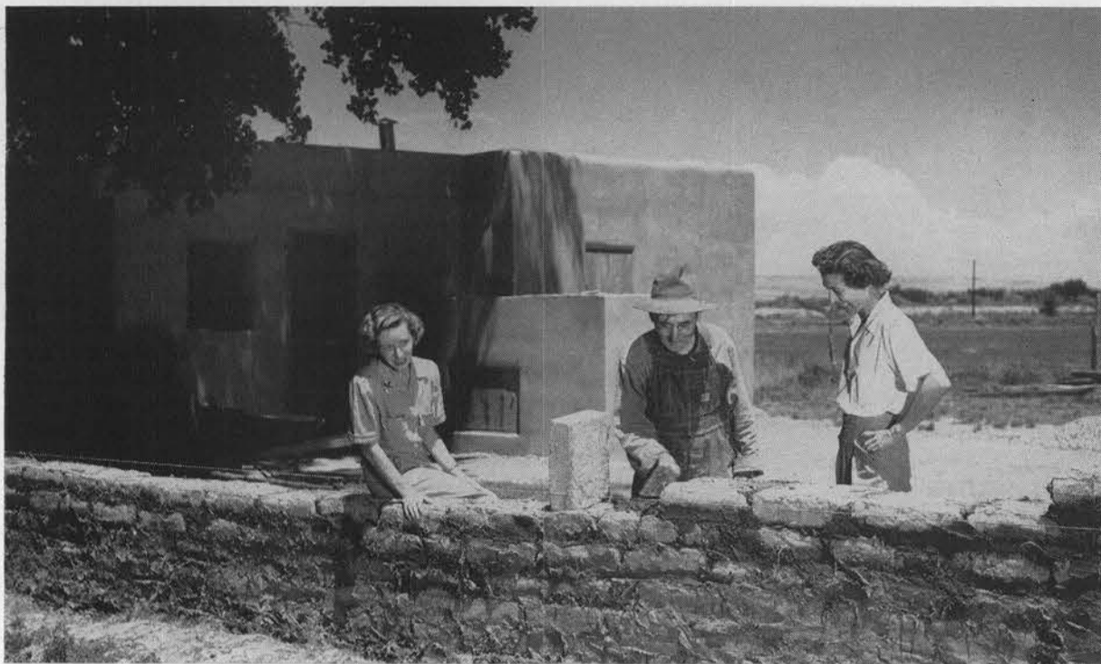
THREE-YEAR PLAN for improving their dream home in the valley includes this adobe wall. Kay Norton, left, and Dorothee Drury, right, watch Billy Lester lay the bricks the same as the original walls of the house were built more than 125 years ago. Much of the work on the home is being done by the girls themselves; they even do the heavy jobs of laying building blocks and raising roof beams.
