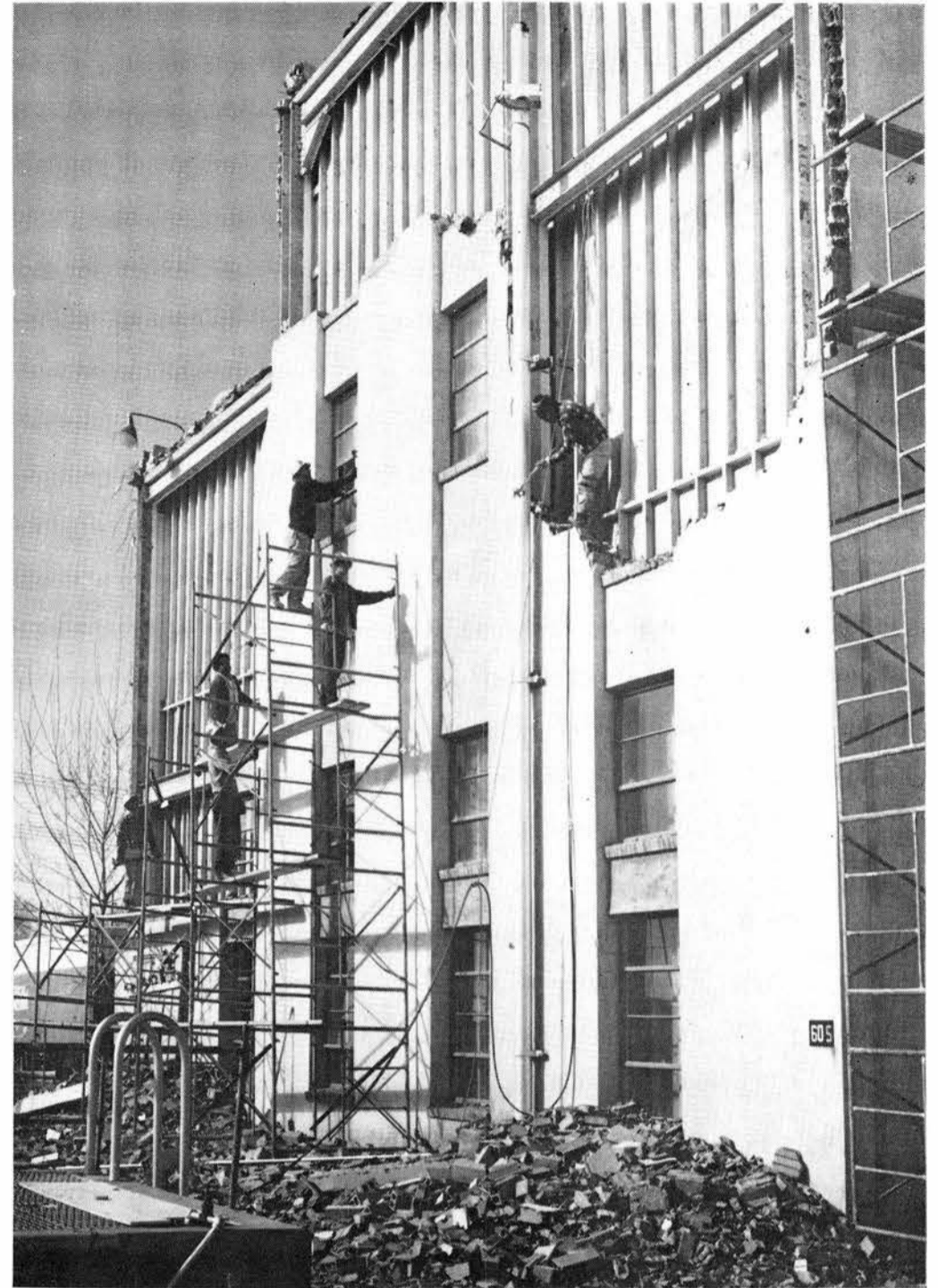
MAKING WAY for a new addition to Sandia Laboratory's steam plant, workmen remove the east wall of the existing building. The project will add 161,000 cu. ft. of space to the three-story steam plant to house a new 1000-lb.-per-hour steam generator. Also installed will be a 5000-barrel fuel oil storage tank and transfer facilities. Total cost of the project will be $815,000. Completion is expected about Sept. 1, according to Plant Engineering project engineer Carl G. Whitcomb.
