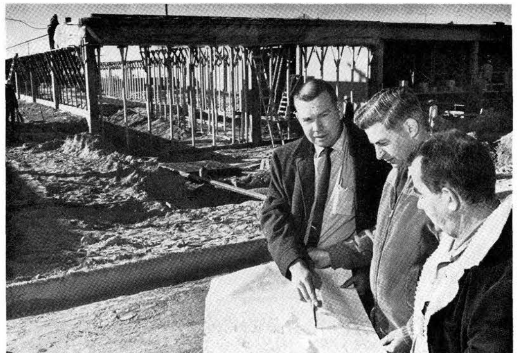
NEW ADDITION to the east side of Bldg. 880 is about 15 percent complete. C. N. Morrisett (left) and Tom Eglinton, project engineers with Building and Facilities Design Division II 4543, checked progress last week with Don Payne (right), construction company superintendent. The 22,500-square-foot addition will house new Sandia computing facilities.
