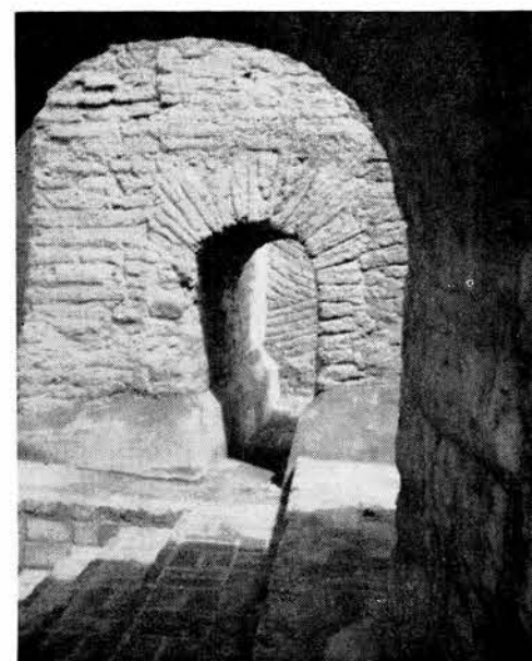
DOUBLE ARCHES within the Pecos mission church illustrate the intricate brick work of the original structure. The stone floor has been re-mortared since the site became a national monument.
