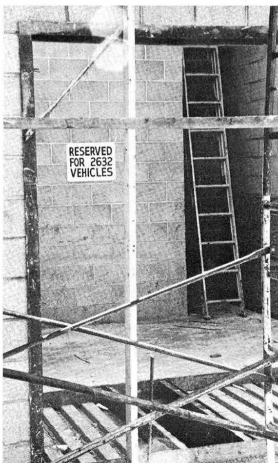
SIGN posted inside small utility addition being built on the northeast side of Bldg. 880—maybe they'll shrink them to Goldfinger-type cubes for stacking?
