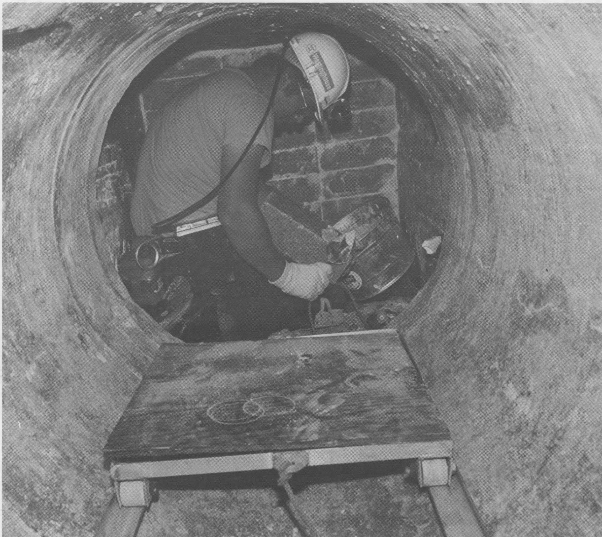
SALT BLOCKS, made underground with a special machine, are the key element in one proposed method of sealing shafts and horizontal bores after wastes are in place. Here, a Westinghouse worker applies a salt-dust paste to a block before setting it in place in a horizontal test drift. (Westinghouse photo)
