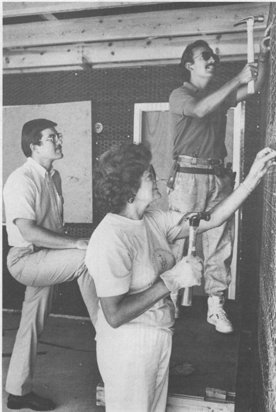
SANDIANS VOLUNTEER their time to rehabilitate old houses or build new ones for low-income families through Habitat for Humanity. Putting up chicken wire in preparation for stuccoing are (from left) Chris Rautman (6315), Margaret Chavez (5211), and Lupe Arguello (1521).
