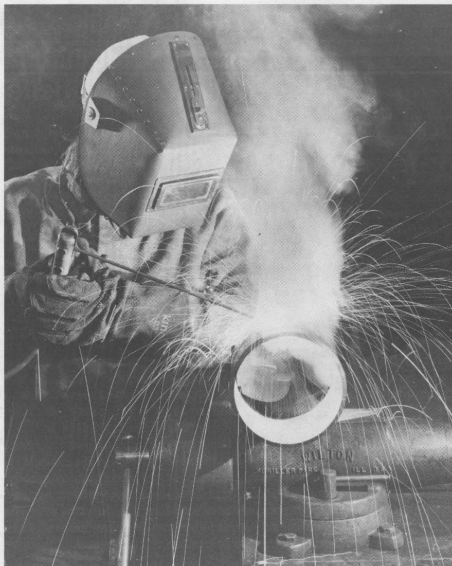
MASKED MAN ROBERT SILVA (7813), pipe fitter apprentice, seals a pipe joint as part of his hands-on training at Sandia. During their five-year apprenticeships, trainees spend 10 percent of their time in formal classroom instruction and the other 90 percent doing hands-on work under an experienced journeyman. Apprentice programs at Sandia, one in Facilities Org. 7800 and three in Materials Process Engineering and Fabrication Org. 7400, have provided training in the major trades since 1958. (Photo by Randy Montoya, 3162)
