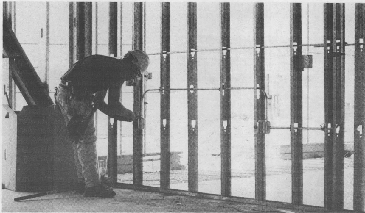
WIRED — An electrician installs wiring in the Integrated Manufacturing Design Facility (IMDF). An average of 700 construction workers are on site every day at Sandia.
