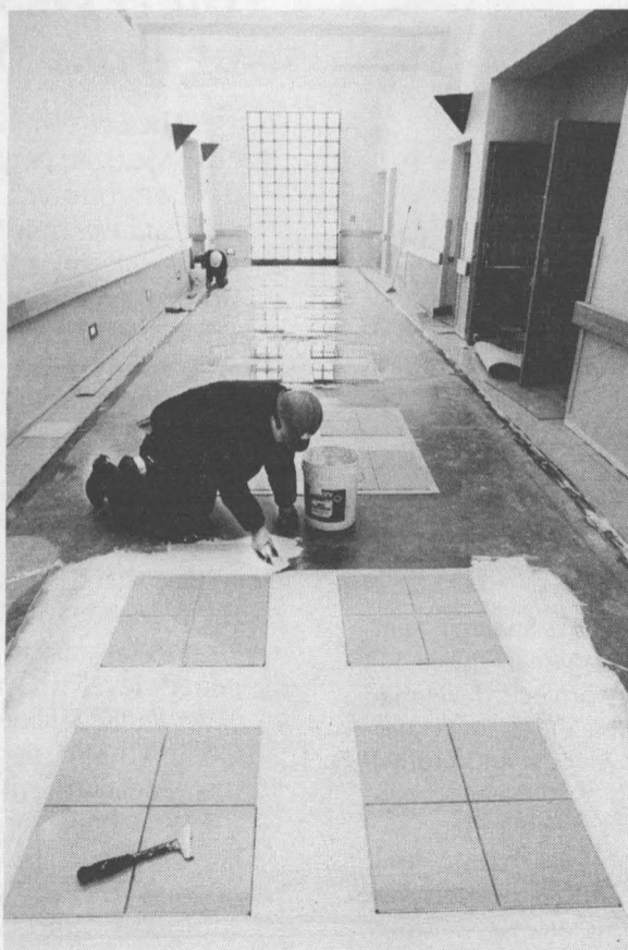
TILE TIME — Jimmy Lujan of Business Environments lays tile in the new Center for National Security and Arms Control (CNSAC) building, a four-story facility expected to be occupied in 1996.
