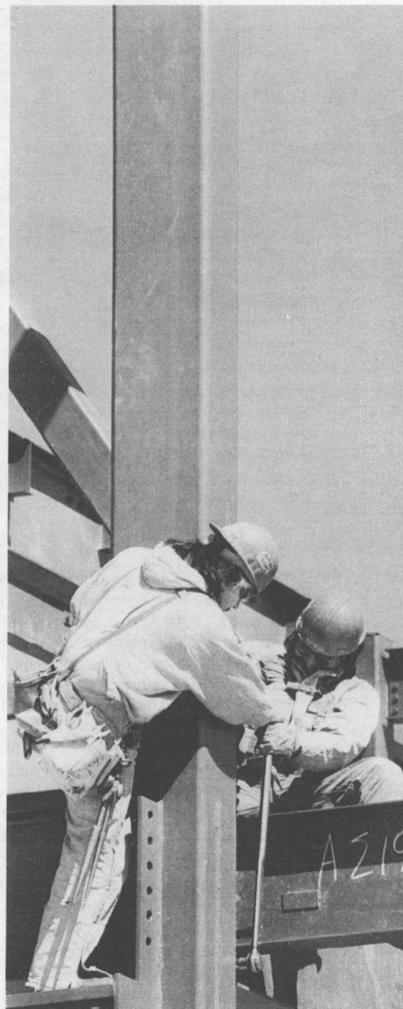
BEAM ME UP — Steelworkers tighten bolts at the two-story RMSEL. Completion of the RMSEL is scheduled for January 1997.
