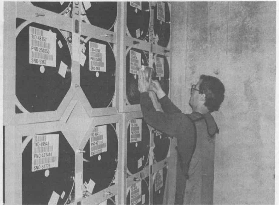
HANDS-ON — Brad Mickelsen (5371) installs sensors inside a storage magazine at the Pantex Plant. They provide continuous monitoring of the room.
